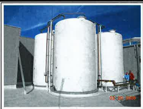
10' Diameter Vertical Chemical Storage Tanks
