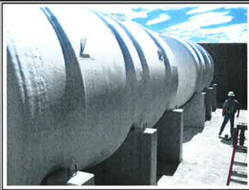
10' Diameter Horizontal Chemical Storage Tanks
