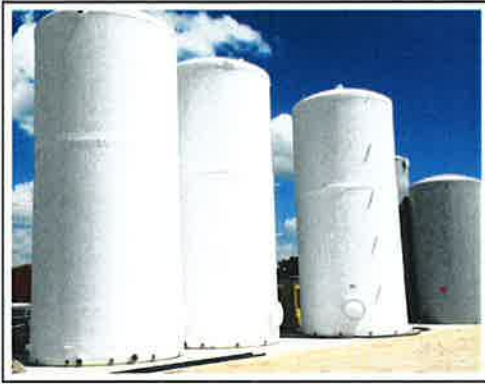
14' Diameter Vertical Chemical Storage Tanks
