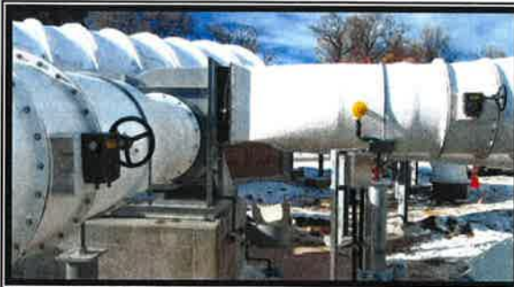
Spunstrand Product at a Water Reclamation Facility
