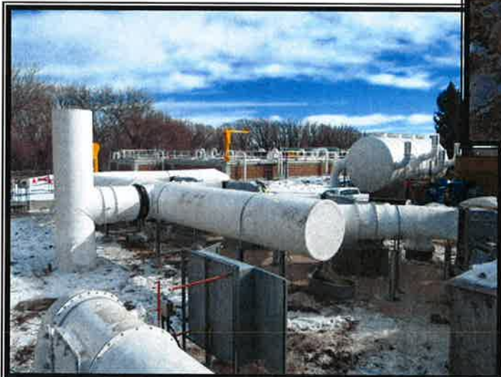
Spunstrand Product at a Water Reclamation Facility
