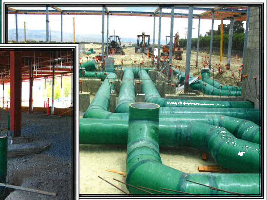
Custom Installation Under an Art Gallery
