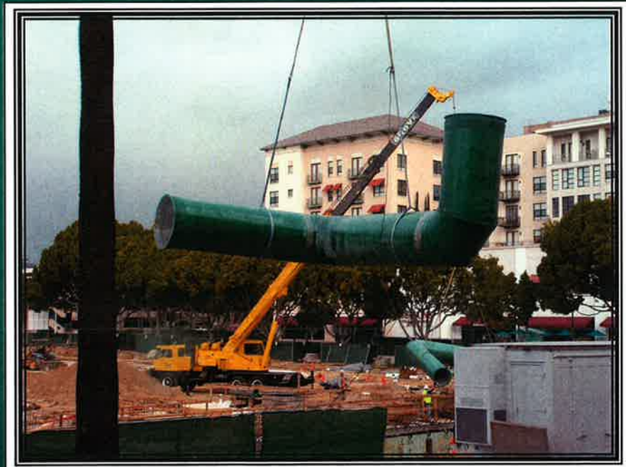
Large Manifolder Sections Available Convention Center
