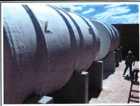
10' Diameter Horizontal Chemical Storage Tanks
