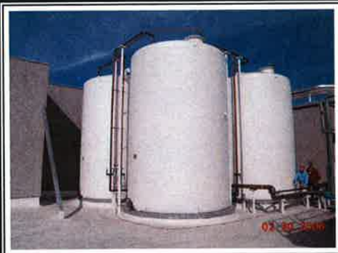
10' Diameter Vertical Chemical Storage Tanks
