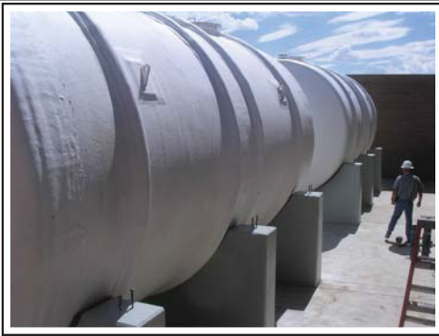
10' Diameter Horizontal Chemical Storage Tanks
