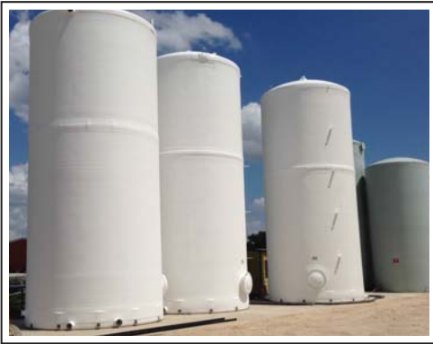
14' Diameter Vertical Chemical Storage Tanks
