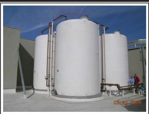
10' Diameter Vertical Chemical Storage Tanks
